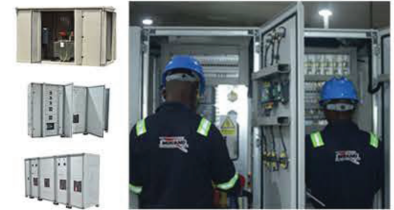
Customized Panels and Compound Sub Station built by Mikano
