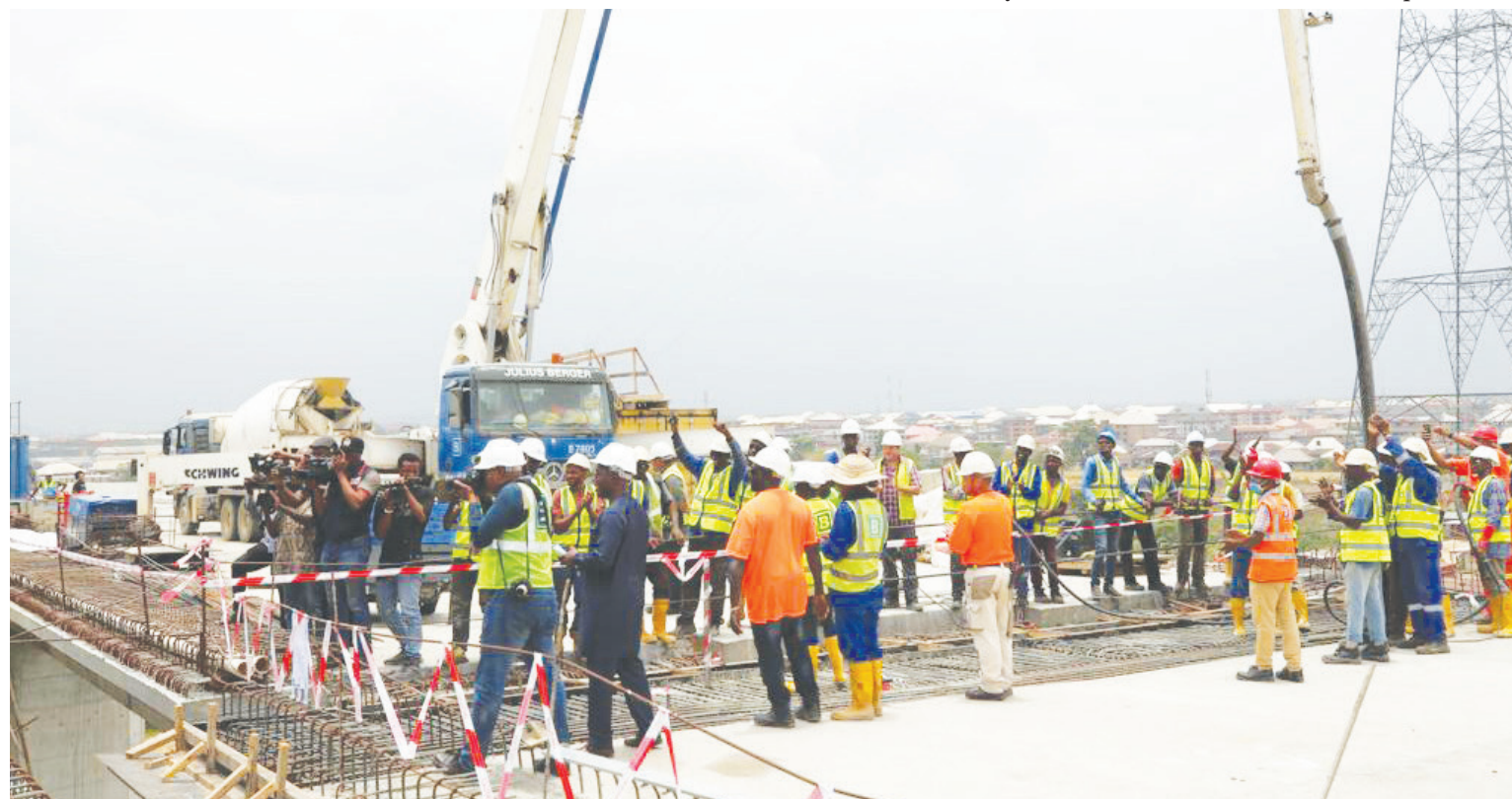
● Workers on site preparing for the flooring of concrete on the bridge.
