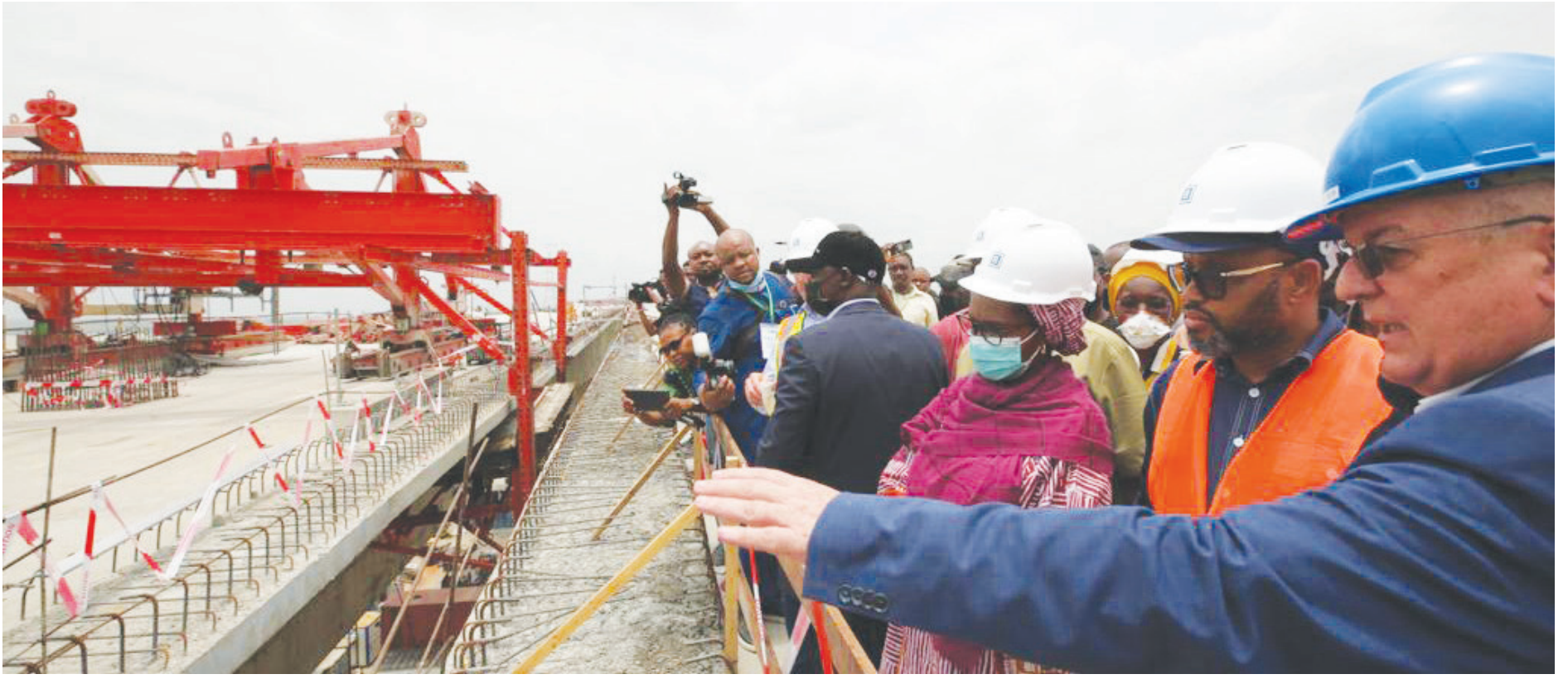
● The Honourable Minister of Finance, Budget & National Planning, Mrs. Zainab Ahmed, with Dr. Gilbert Ibezim (middle), and Mr. Fredrich Weiser, Project Director, Julius Berger at the site explaining the flooring of concrete on the final segment on the super structure of the 2nd Niger Bridge.
